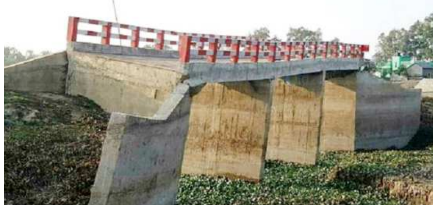
This bridge, tilted just before inauguration, at Nirail village in Tangail's Basail upazila has not been repaired in five years, much to the suffering of local people. PHOTO: STAR
