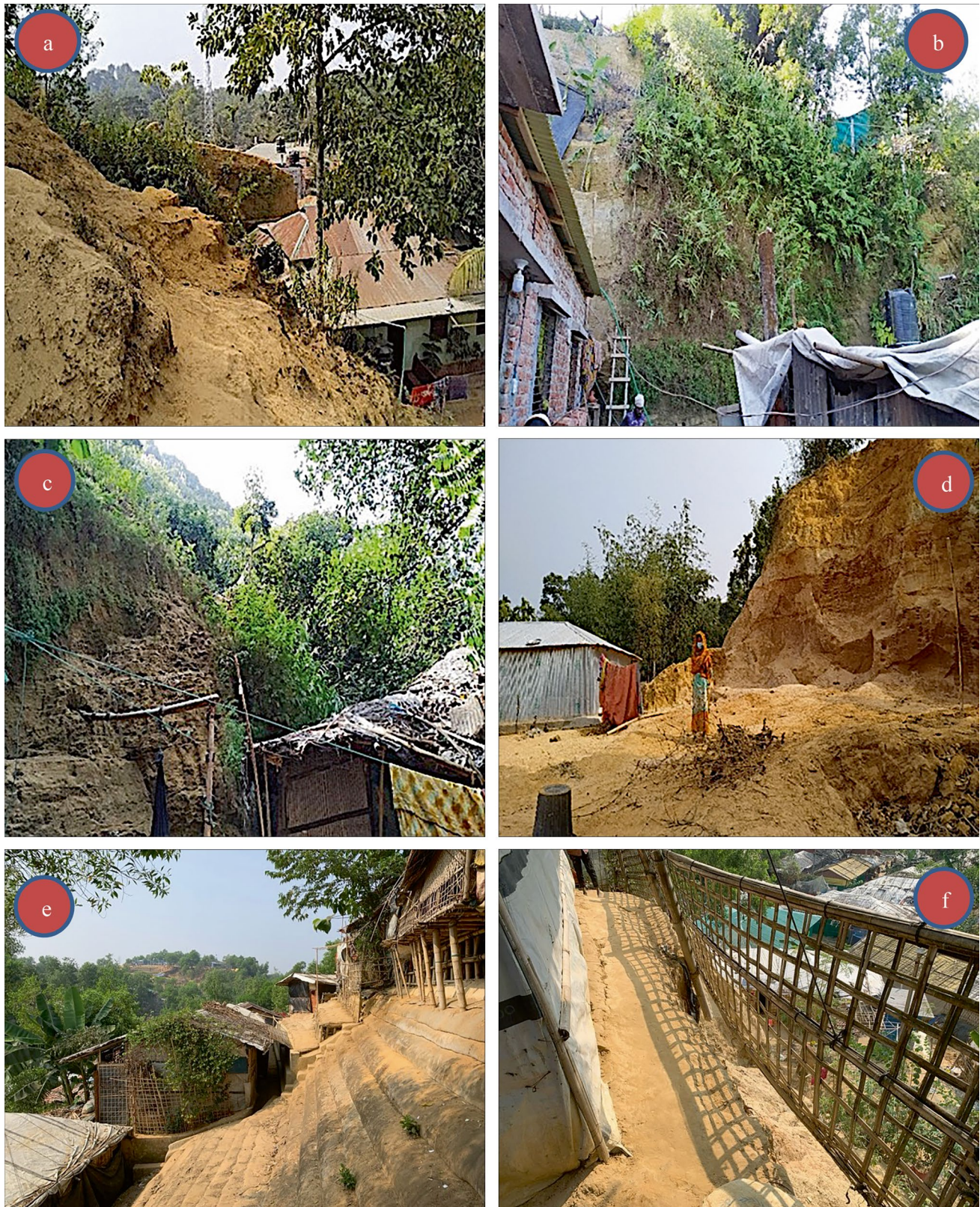
Fig. 4 Landslide vulnerable houses located on the (a, b) urbanised and (c, d) rural hilly communities, and (e, f) the Rohingya refugee camps in Cox's Bazar district. (Source: The authors, fieldwork, 2021 and 2023)
